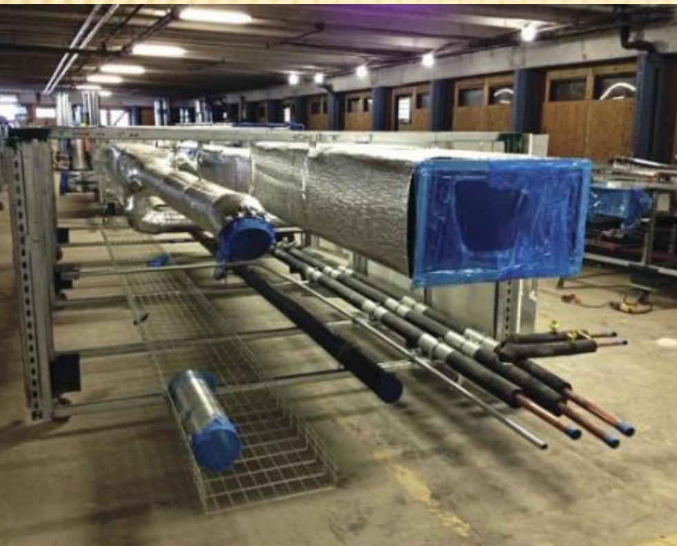
MEP Corridor Racks
