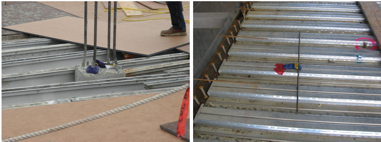
Figure A12.3: Concrete strap attached to column reinforcement (left), and floor reinforcement (right)
