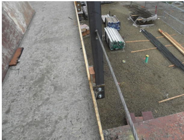
Figure A12.1: Guardrail attached to concrete imbeds at the edge of the concrete slab
