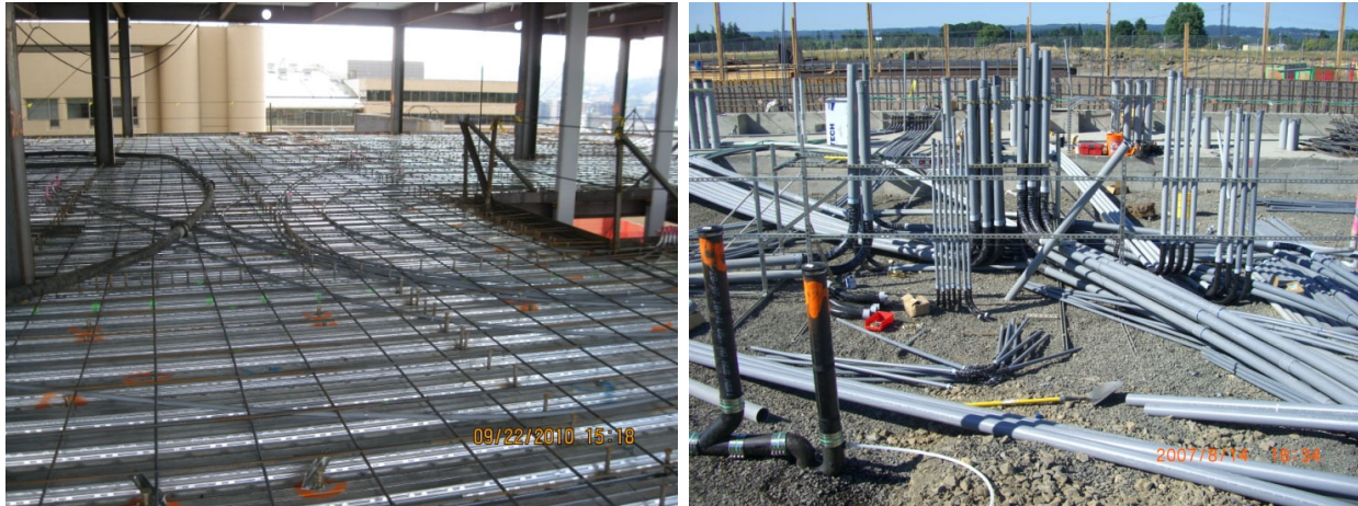
Figure A12.7: Electrical wiring placed in the floor before casting (left), and at foundation level (right)
