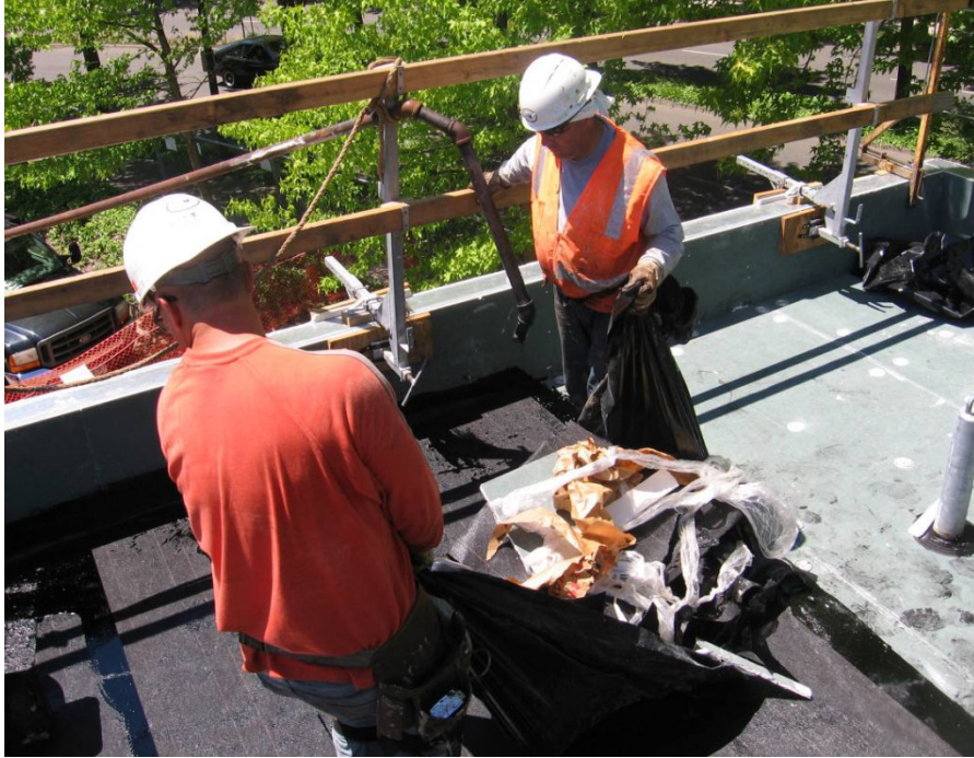
Figure A12.9: Construction workers placing insulation on the roof (Rajendran and Gambatese 2013)
