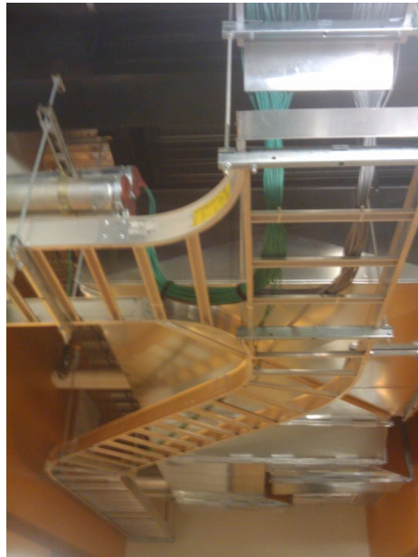
Figure A12.6: Electrical cables running in conduit and on cable trays
