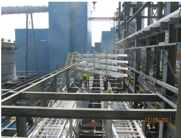
Figure A12.10: Cable tray being lifted into place (Picture provided by URS Corp.)
