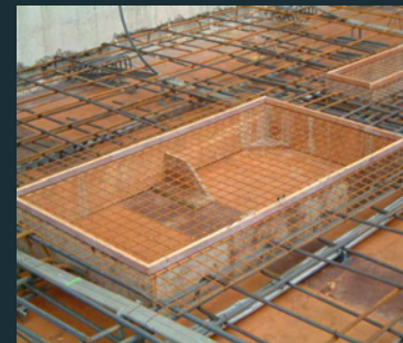
3. Small metal mesh prevents falls in open areas
